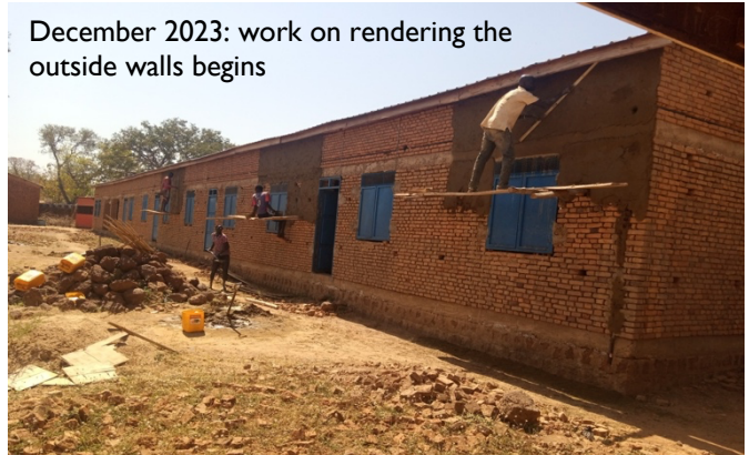
2024: windows already in place, work on laying the concrete floors is under way
