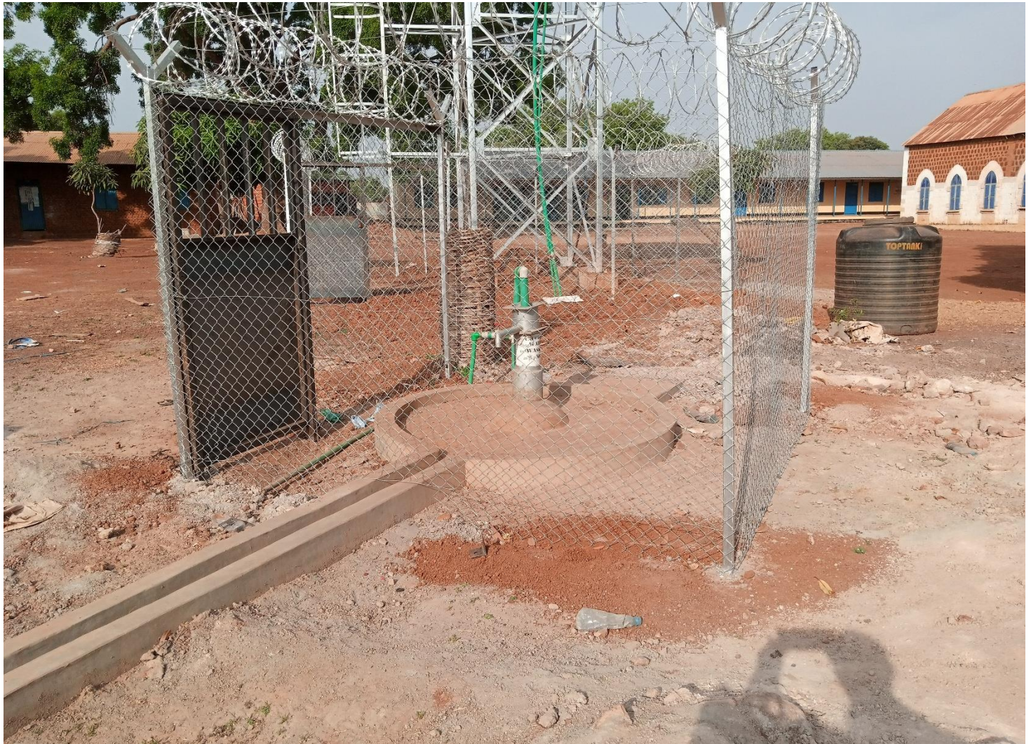
Figure 7: Bore Hole and the fence with security wires on 28/12/2025.
